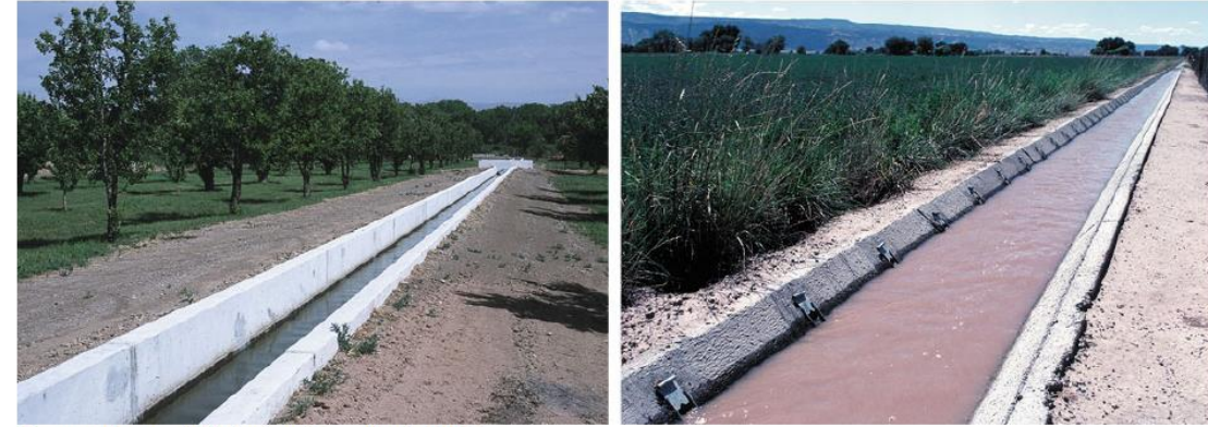
Square and trapezoidal irrigation ditches (Credit NRCS)
